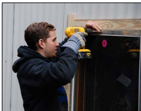
Documenting "WorkFest 2008" when close to 500 students from 43 colleges gave up their Spring Break to repair and rebuild 24 homes for needy families.
