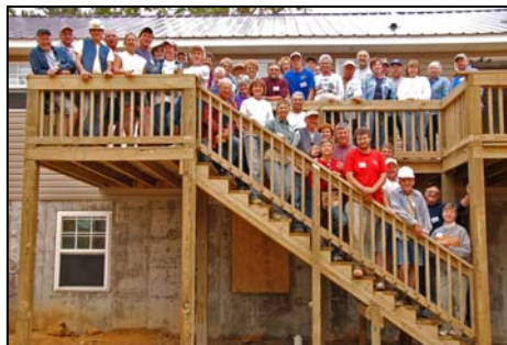
The construction of a new home, in six days, by 43 members of the Fox Valley Mission Group from Wisconsin for a Kentucky family with three disabled family members.
